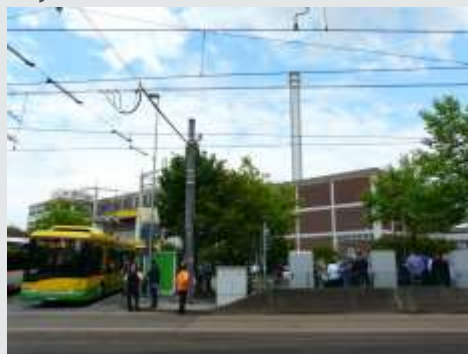
Fig 11: Charging station for electric bus and electric cars powered from tram overhead line in Oberhausen, Germany.
