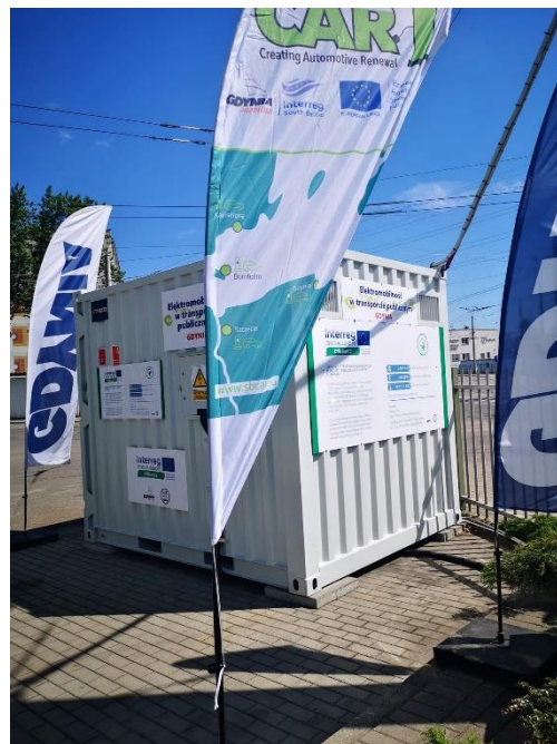
6. Figure: Energy inverter in Gdynia, Poland to use or recuperated braking energy (source: PKT)
