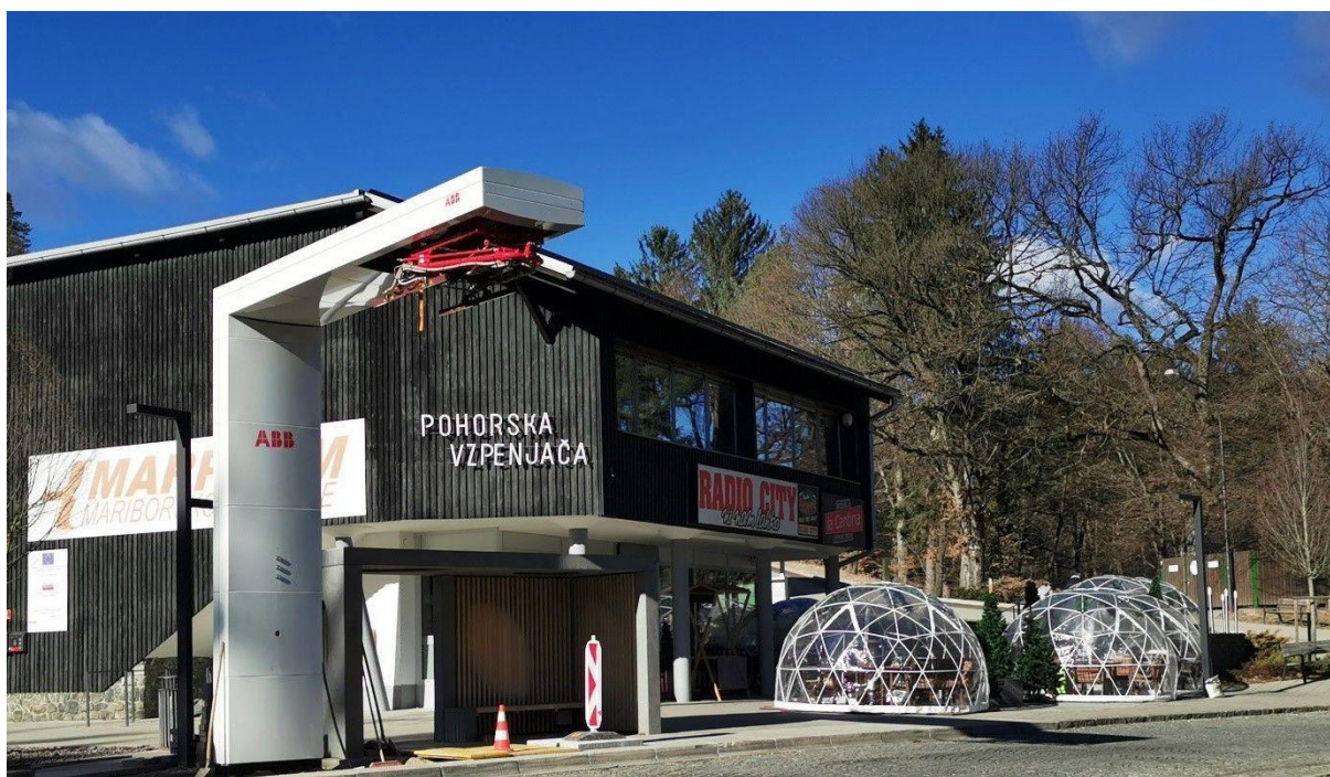
14. Figure: E-bus fast charger in Maribor (source: Municipality of Maribor)
