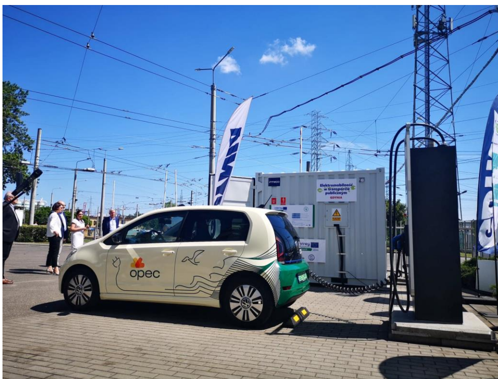
7. Figure: The energy inverter connected to an electric charging station (source: PKT)
